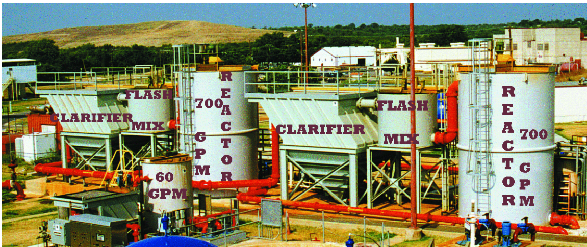
Figure 1. Co-precipitation system (1-60 gpm and 2-700 gpm) installed by SAIC
